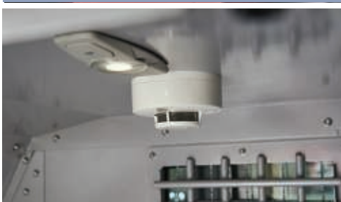
Dome light and smoke detector
