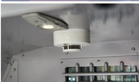
Dome light and smoke detector
